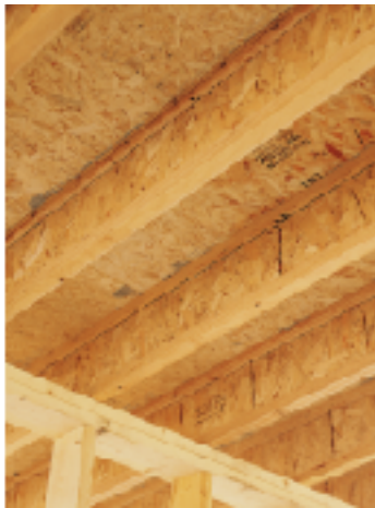
Engineered wood I-joists and OSB subflooring.
